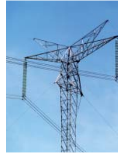
Furnas 600 kV ±DC
